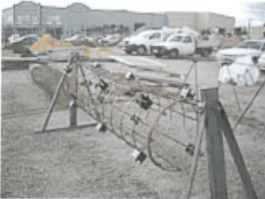
Western power substation Kewdale
